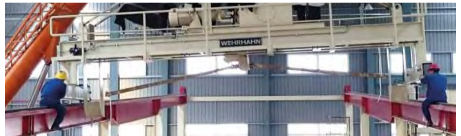
Installation of the last machines at Baopeng in China
