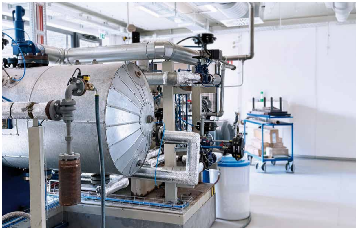
In the autoclave AAC blocks or fibre cement sheets are steam cured.
