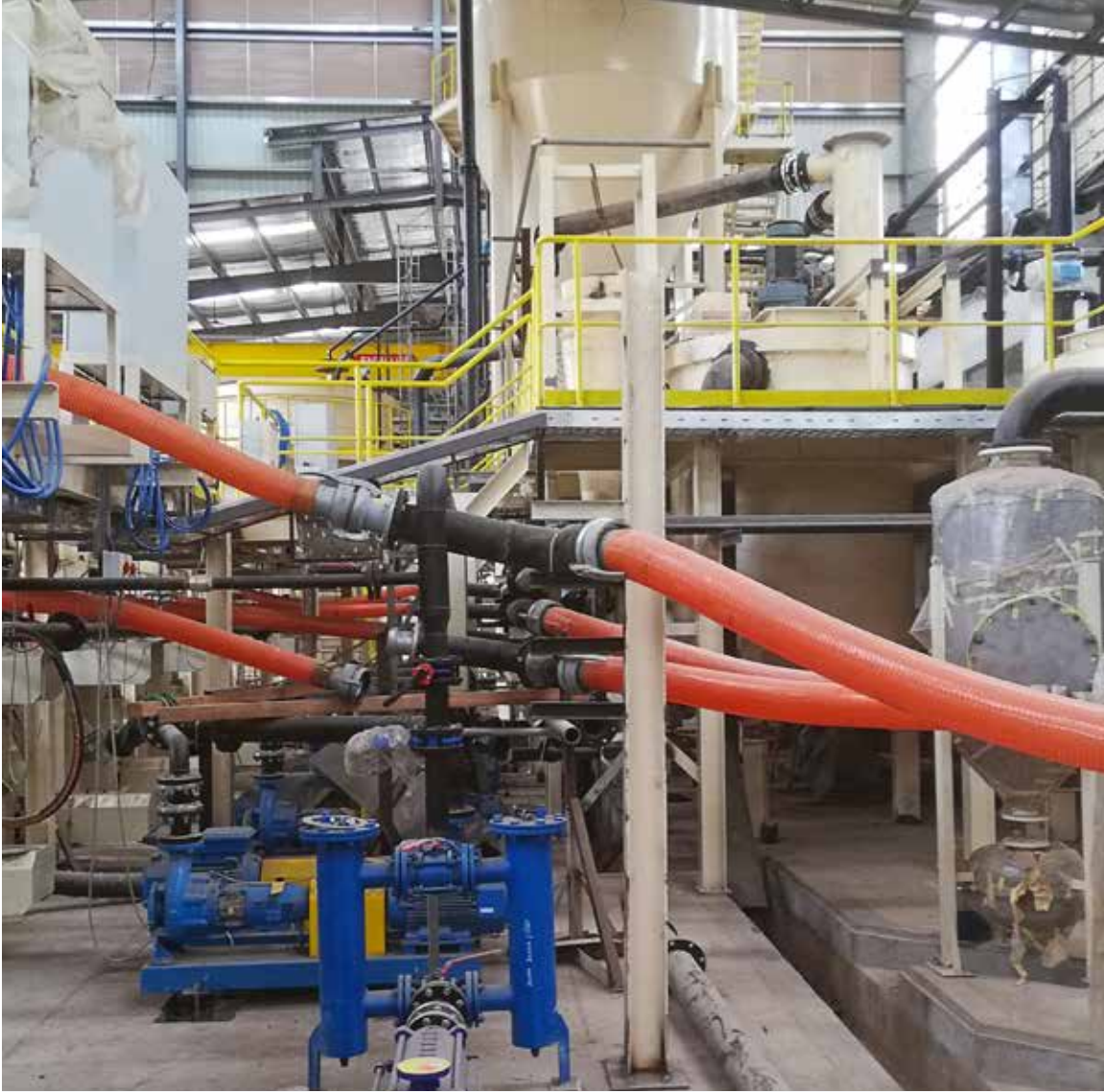
Great progress: Despite difficult weather conditions in Sri Lanka, the installation team cannot be held back!
